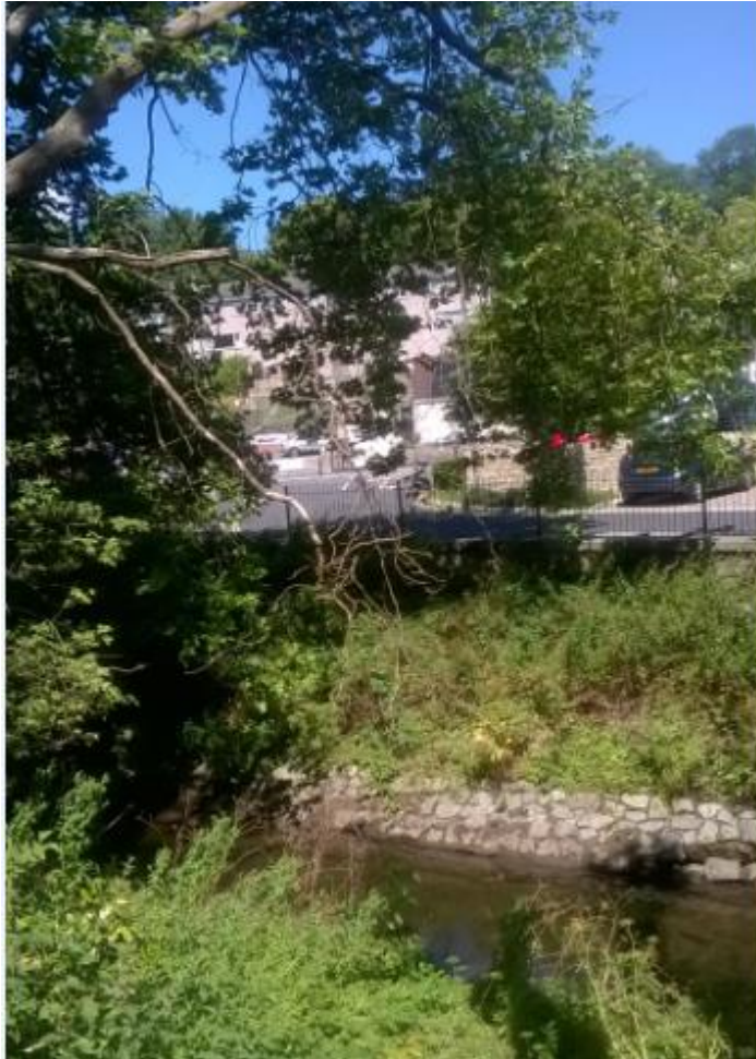
The revetment requiring repair
